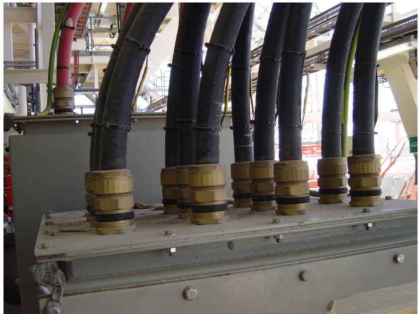
Figure 207: Flameproof cable glands installed on an enclosure
